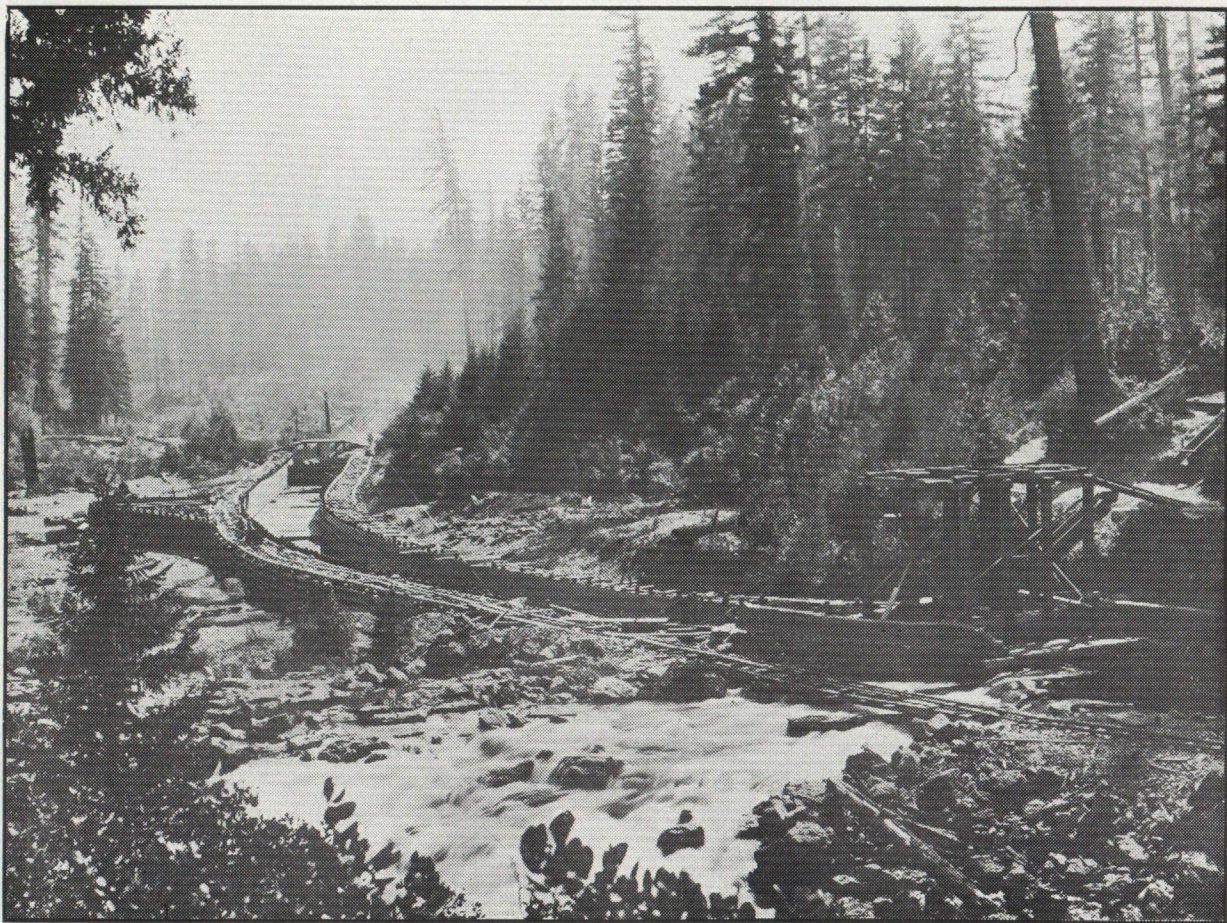
INTAKE OF FLUME FOR PROSPECT POWER PLANT WHERE A MILLION DOLLARS IS BEING SPENT DEVELOPING 50,000 HORSEPOWER FOR USE IN MINES AND FACTORIES OF SOUTHERN OREGON
