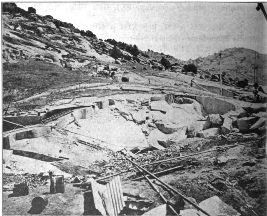
Number 1 Quarry of California Granite Company, situated 4 miles east of Porterville. Photo by Walter W. Bradley.
