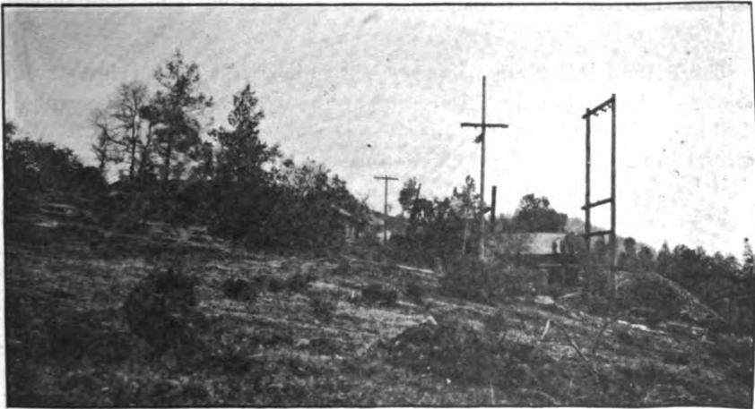
Photo No. 13.—Hoist and transformers at the Banner quartz mine south of Monte de Oro and four miles northeast of Oroville.
